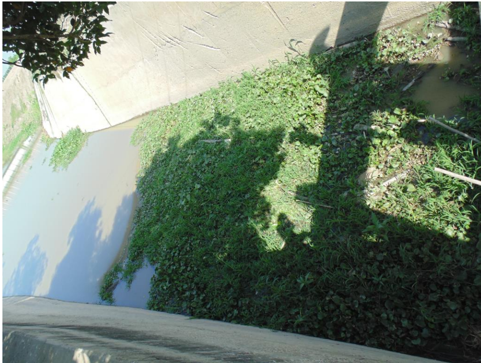
Photo 3: Faulty or insufficient maintenance of the input gate freshwater down the piper de aguas negras
