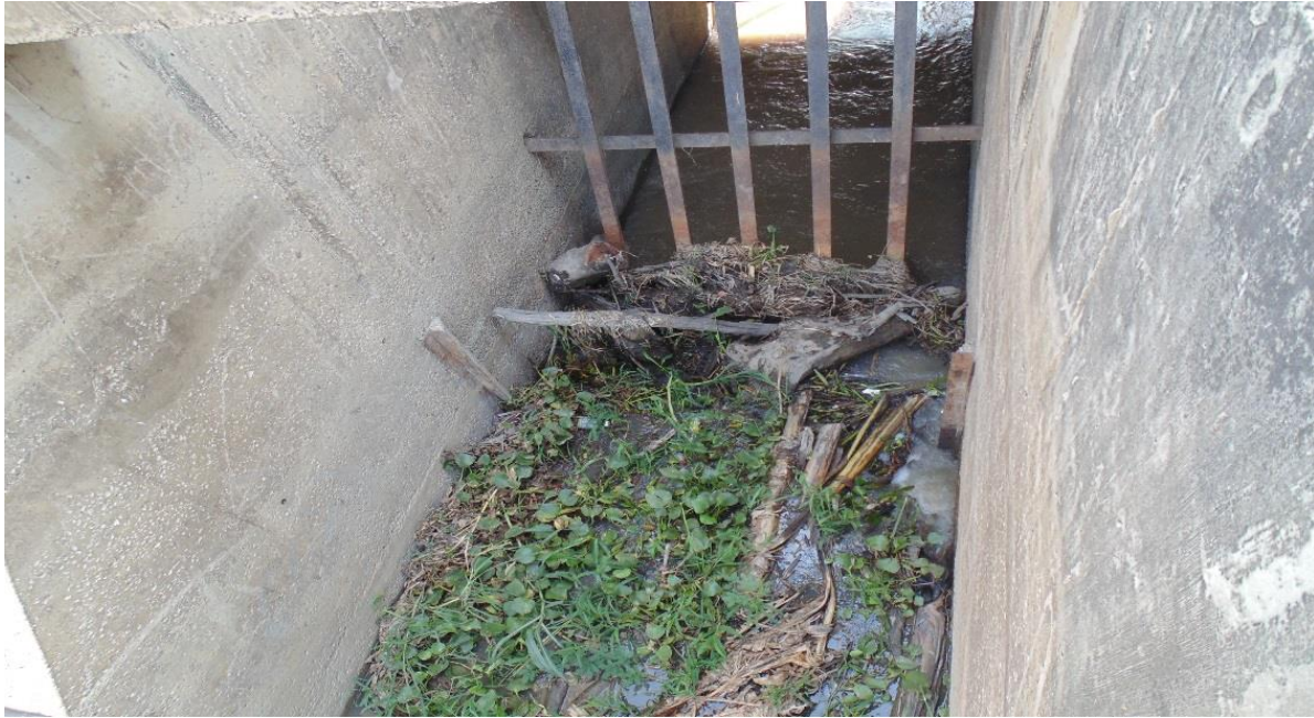
Photo 2: Faulty or insufficient maintenance of the input gate freshwater down the Caño de aguas negras
