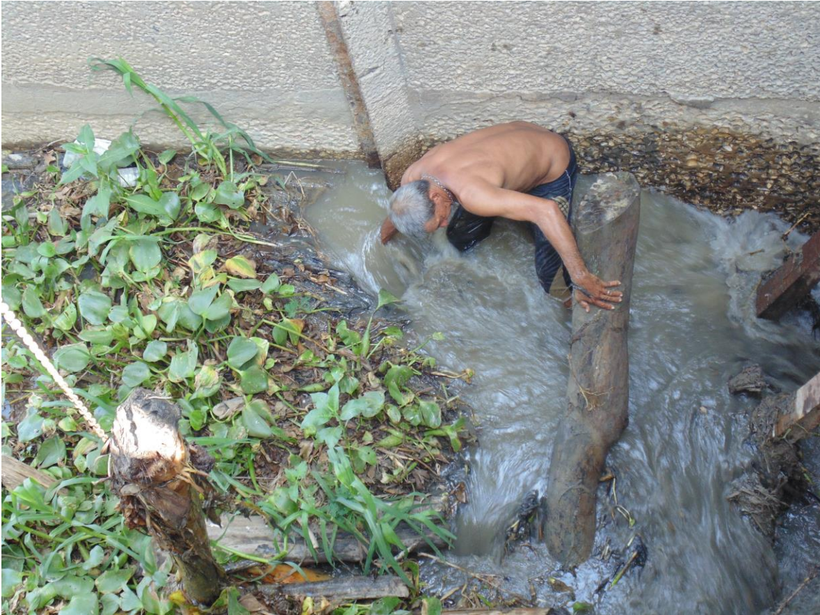
Photo 8: Maintenance handmade by one of the residents of the stilt villages to achieve some freshwater flow to the CGSM
